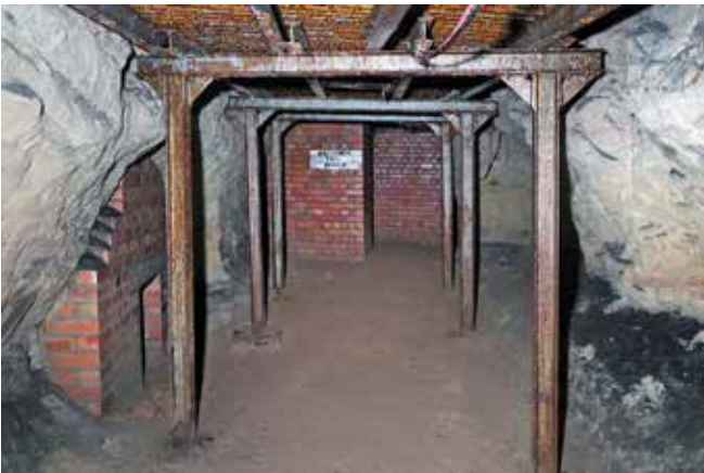
Rouse's Sand Mine: Reinforcement as an air-raid shelter, near Peel Street entrance. Photo Clive Penfold
